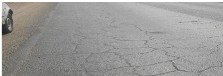
Fig. 2: Fatigue cracking on the pavement
