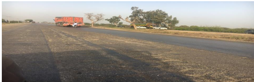
Fig. 1: Pavement distresses observed on Hyderabad - Hala road
