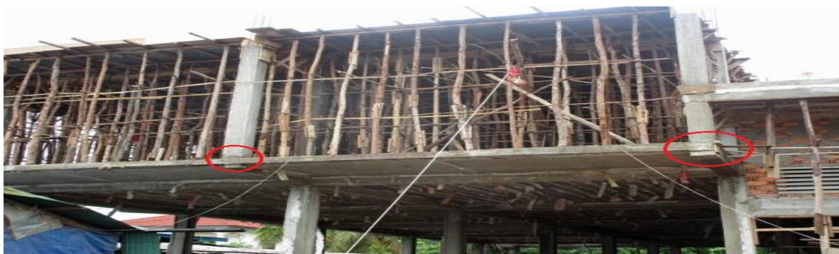
Fig. 1: Red Circle shows Floating Column
